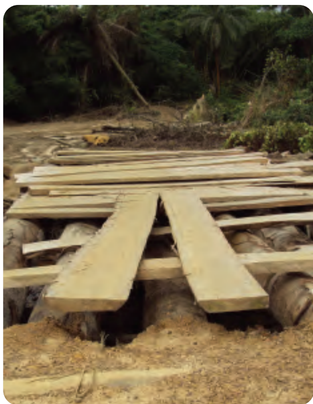
Bridge on logging access road opening up land to forestry. Photo: SDI
